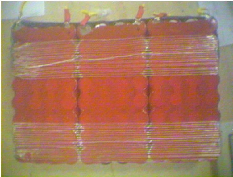
Figure 4-1 42V NiCd Battery Packs (3 of)
